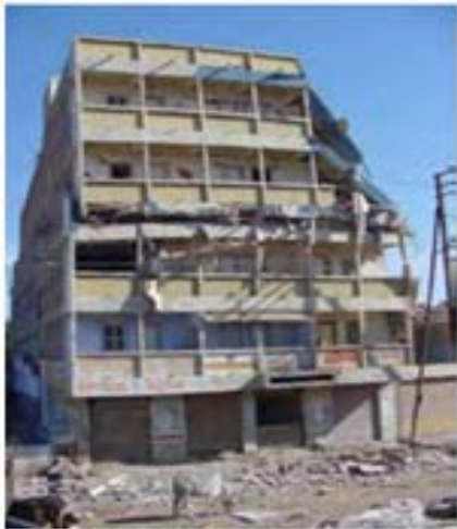
An example of a building collapse due to an intermediate Soft story in the 2001 Bhuj, India -earthquake. Source: EERI 200
